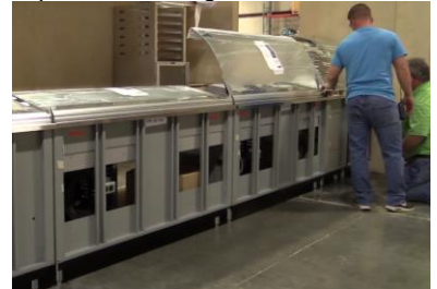
After the first cold unit is adjusted, use it as a baseline to level the rest of the units side to side and front to back.
